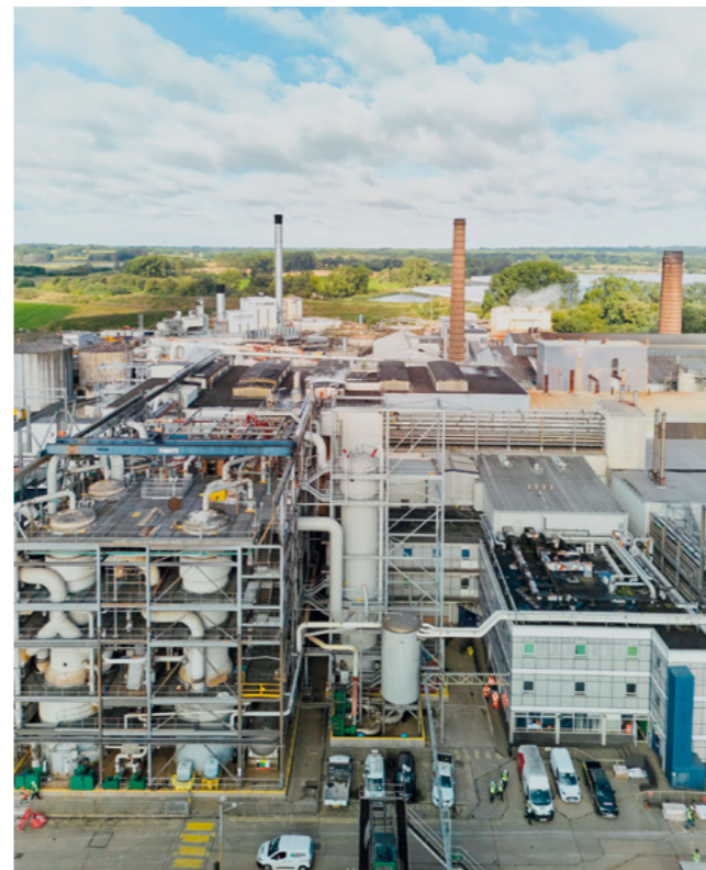
A new evaporator installed at British Sugar's factory in Wigginton as part of a project to reduce site emissions
